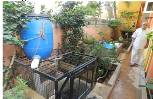
Figure No: 56 Naturally Recharge Wells and Bore Wells
